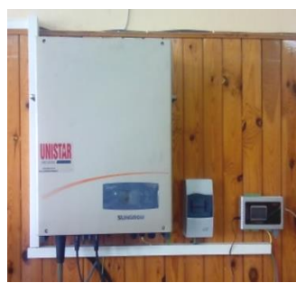
(PV) Grid Inverter Readings
