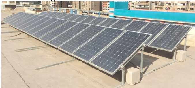
(PV) Panels Modules on Sided/ nearby building Roof
